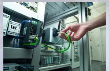
Factory automation PLCs
